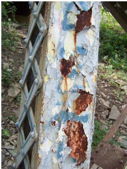
Figure 1. Corroding support of a railroad bridge.
